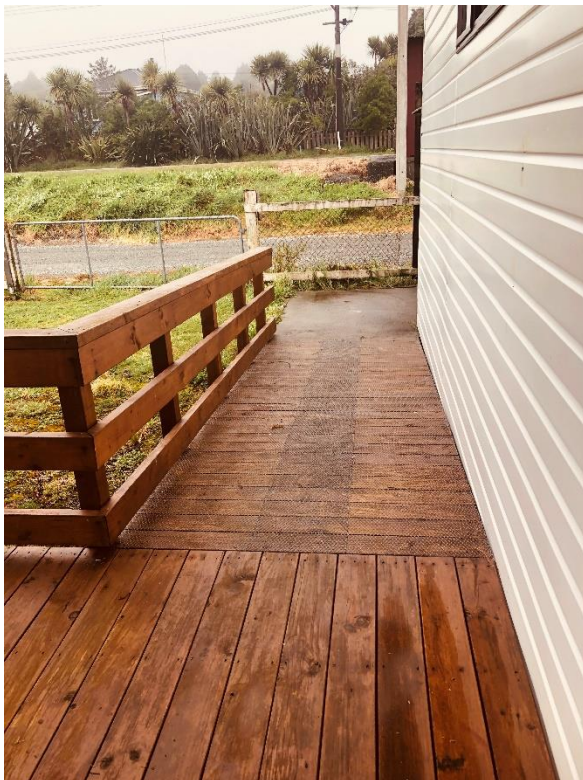
Existing ramp that requires handrails
