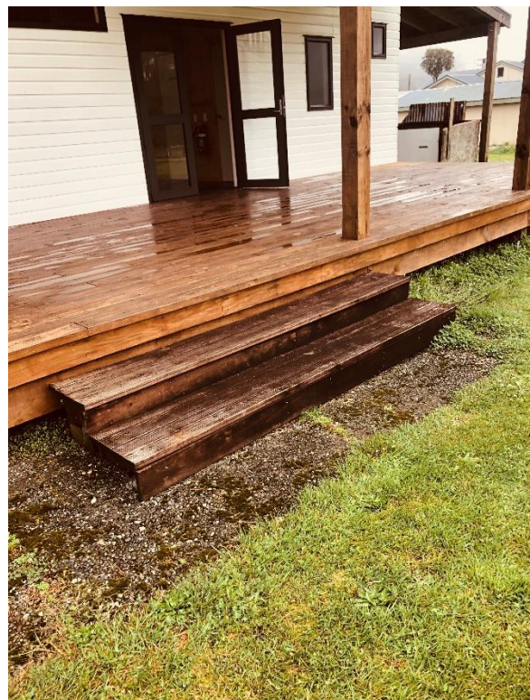
Existing steps to be replaced and requires handrails
