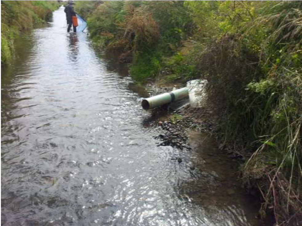
Photo 10: An excavated tile drain outflow pipe, post re-levelling. This drain would not have been operating prior to re-levelling.
